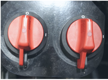
Switches in off position
