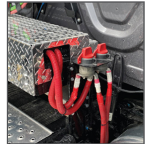
Figure 12. Passenger-side battery disconnects
