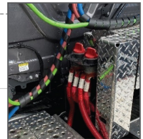
Figure 13. Driver-side battery disconnects
