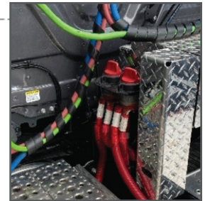
Figure 13. Driver-side battery disconnects
