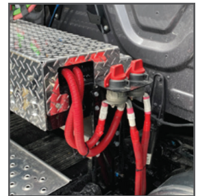
Figure 12. Passenger-side battery disconnects
